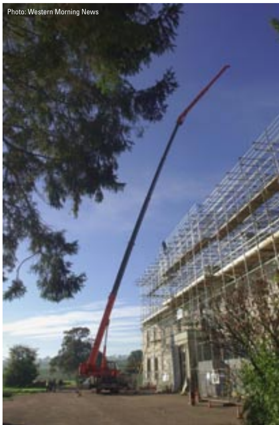
The crane from Apex Scaffolding Ltd lifting the temporary roof protection into place.
